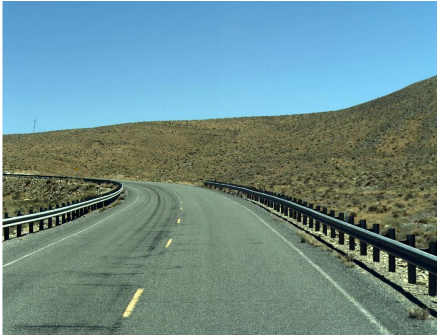
Figure 1. Guardrails on a road
